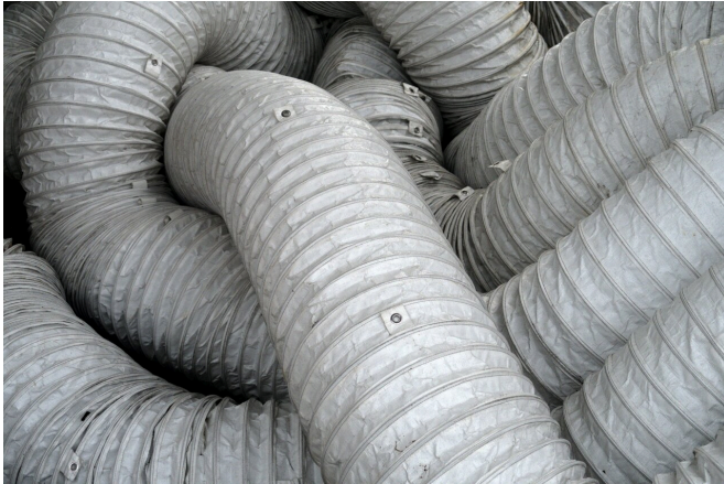
A tangle of ducted air pipes are connected to a portable air unit being used to air condition a large hall. Credit: Martin Visser, Unsplash
